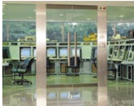
Telekom Control Room.
